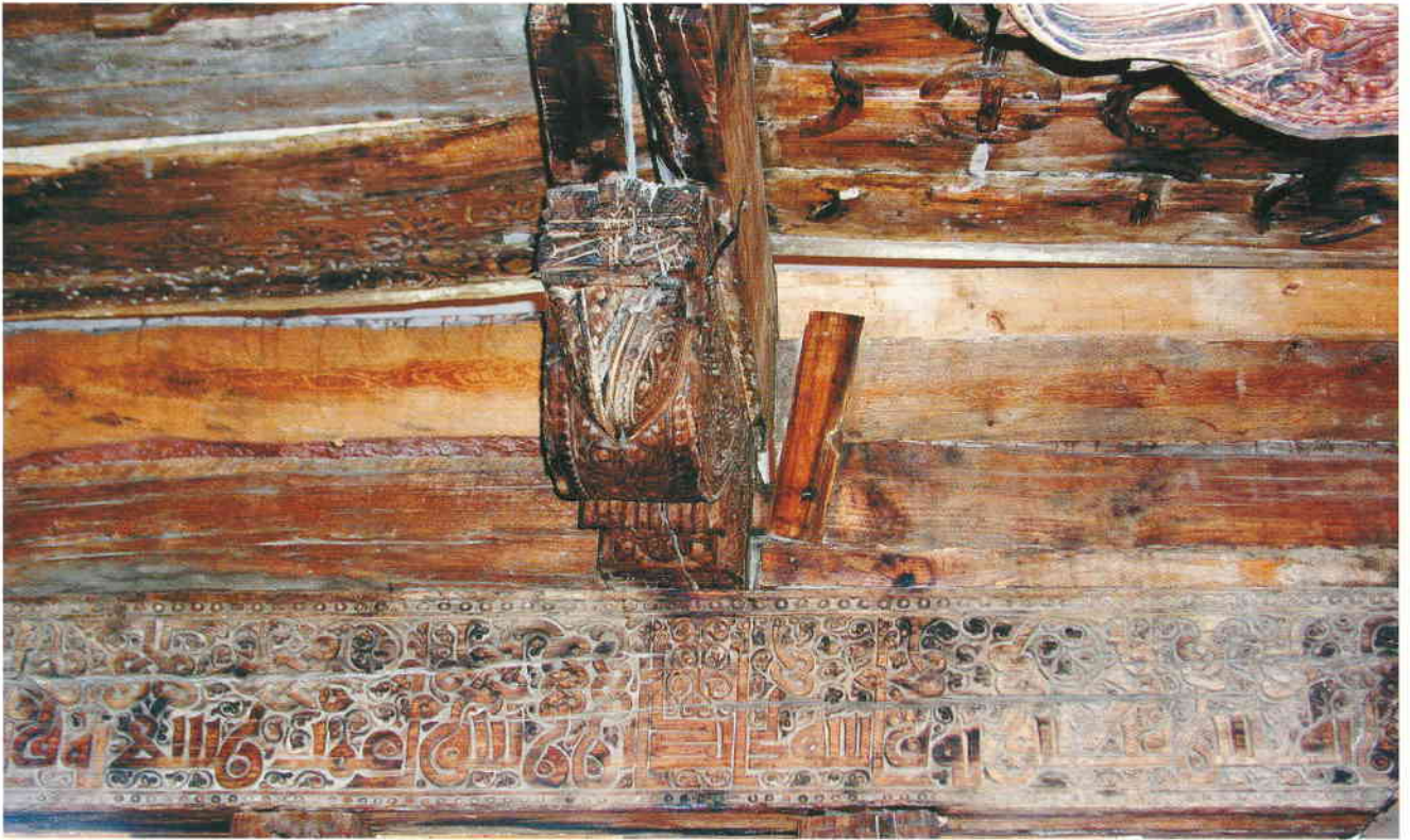
The detail of wooden beam in the Khazrati Shokh mazar. Chorku, 9 th–10 th centuries.
